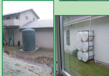
Rainwater catchment systems on Administration Bldg & White House. Total water storage = 18,000 gallons. The prison has decreased the amount of water used per offender from 132 gallons/day (6/03) to 111 gallons/day (6/04).
